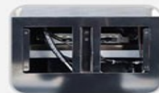
Cable Room Cable hidden interior
